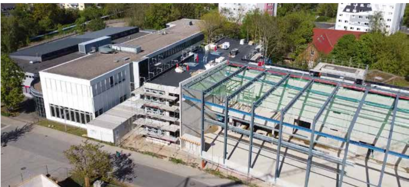
The existing building is on the left. This was built in three construction phases between 2004 and 2013. The construction work for the fourth phase, which can be seen on the right of this image, began in March 2019 and is provisionally scheduled for completion in spring 2021.
